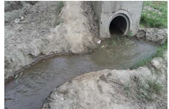
Wastage of water in muddy channels.
