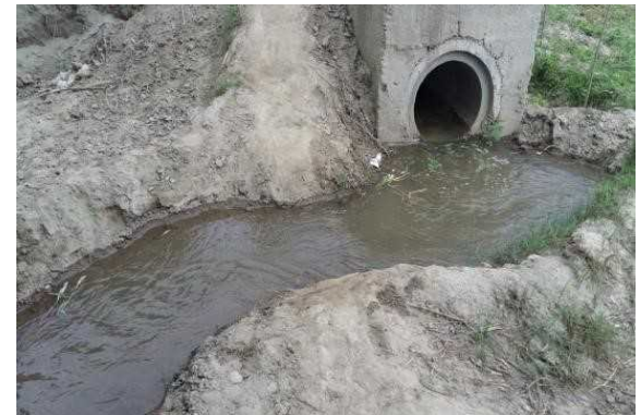
Current situation of water wastage in a muddy channel
