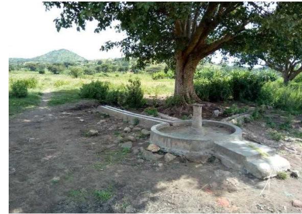
A broken borehole that needs repairs
