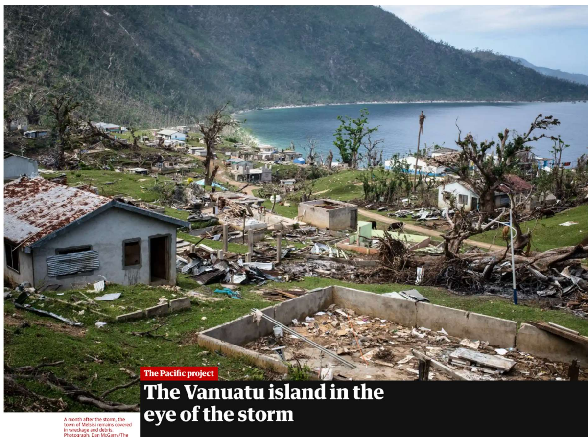
Figure 24 News article showing destruction on Vanuatu's Pentecost Island, including extensive damage to critical WASH infrastructure, in the days after Tropical Cyclone Harold in 2020
