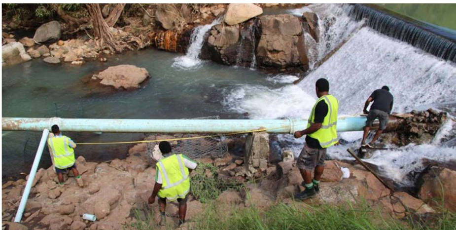
Figure 21 Emergency repairs to water infrastructure undertaken by staff of the Water Authority of Fiji
